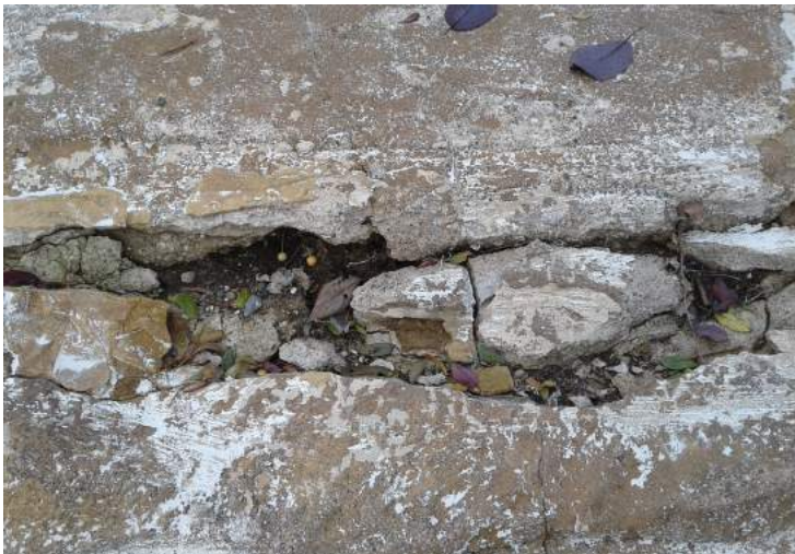
Fully deteriorated sections
