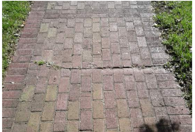
Cracking likely due to significant shifts in paving base
