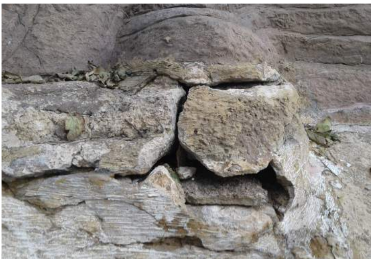
Sections likely to completely fail
