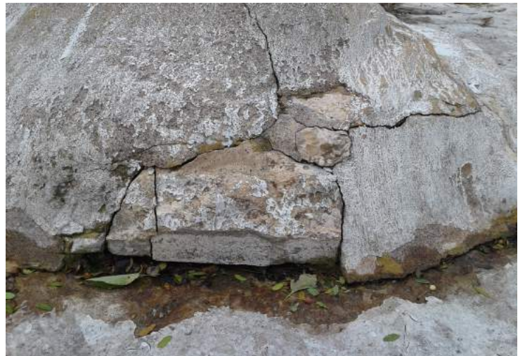
Cracking that suggests likely structural failure
