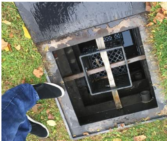
Fountain recirculation return
