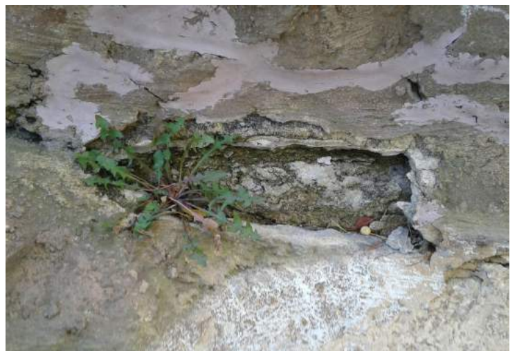
Mis-matched patching and sealing
