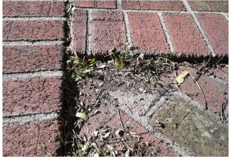
Uneven surface transitions
