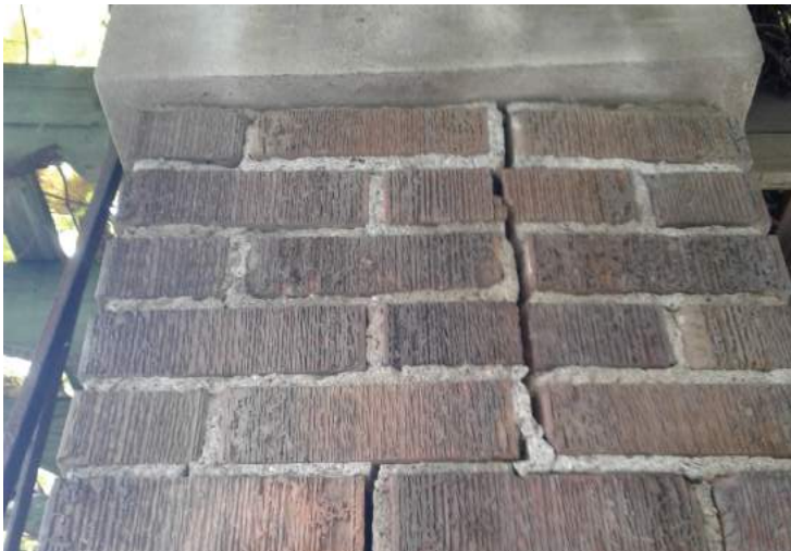
Extensive damage on column 4
