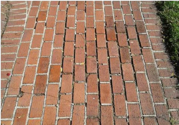
Fully deteriorated mortar joints
