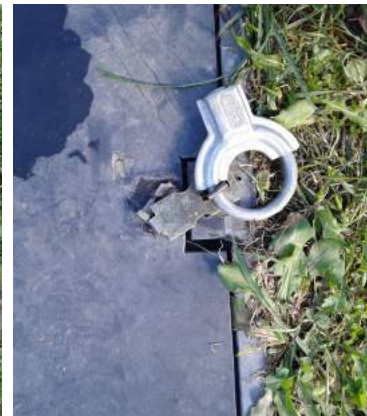
Pump vault lock
