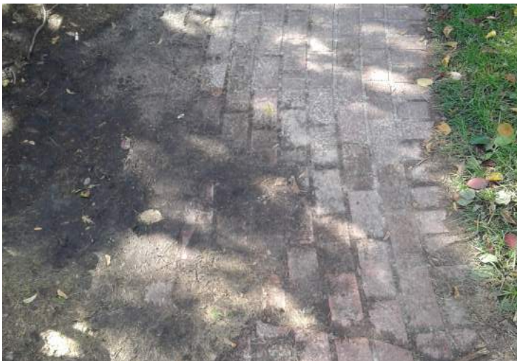
Sand/pooling due to drainage issues
