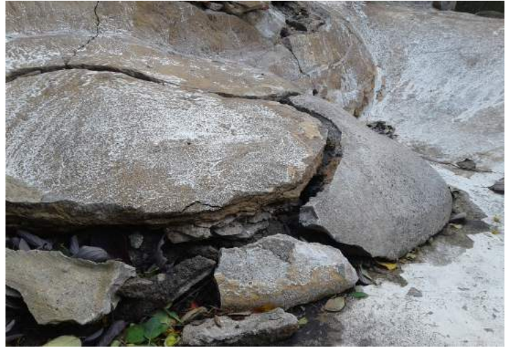
Extensive cracking and broken repairs
